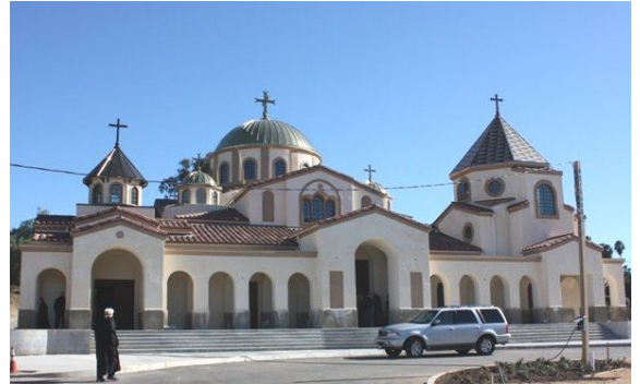
Exterior of St. Andrew Church before the installation of the stone on the walkway and stairs, and the marble wainscoting around the base.
